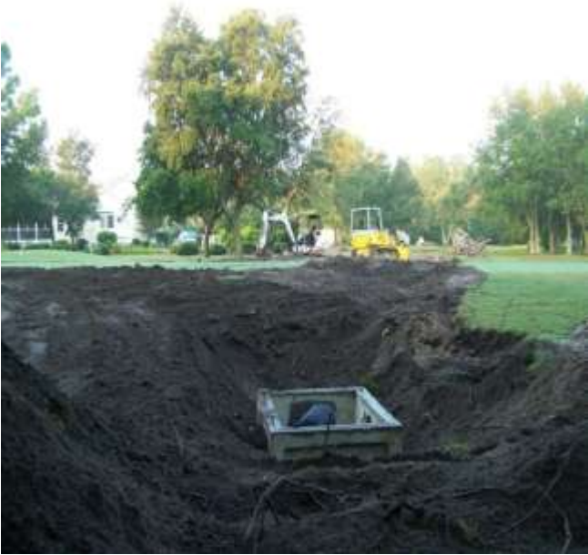
Figure 2--Main three way Junction /Inlet Box @ #4 Tee
