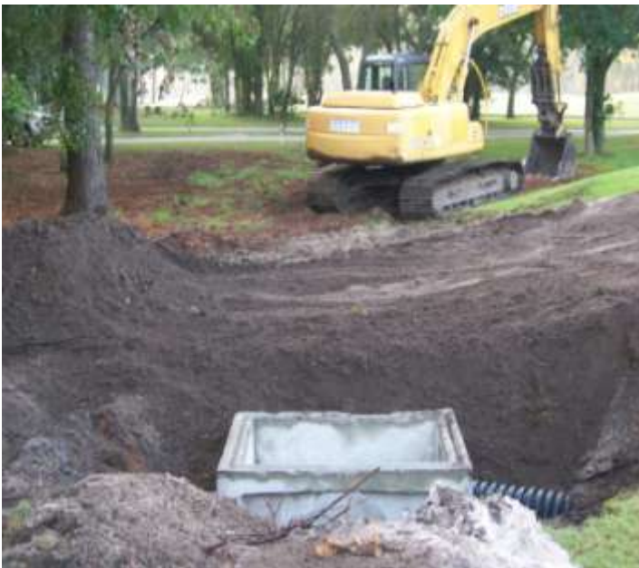
Figure 4-- View from Main J-box toward Marshview Rd.
