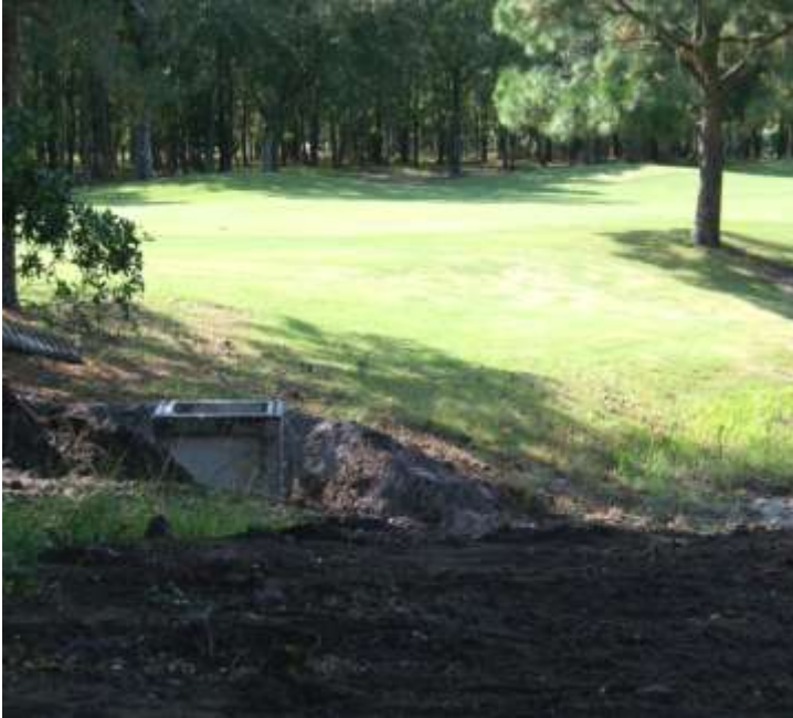
Figure 3---New Pond #20 Control Box
